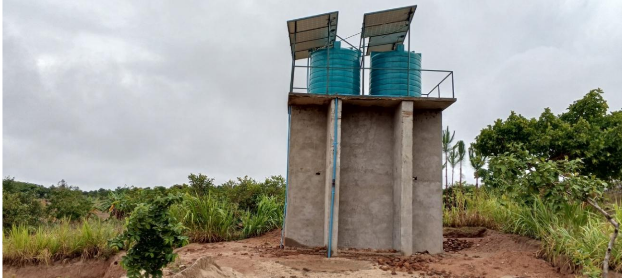
Water tanks for portable access to safe water at APIC
